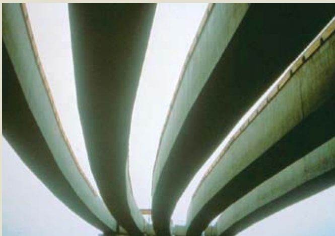
Figure 3. The curved, precast, post-tensioned concrete box girders used for the Philadelphia Airport renovation are in their final position. Courtesy of Joseph Nagle, Schuylkill Co.
