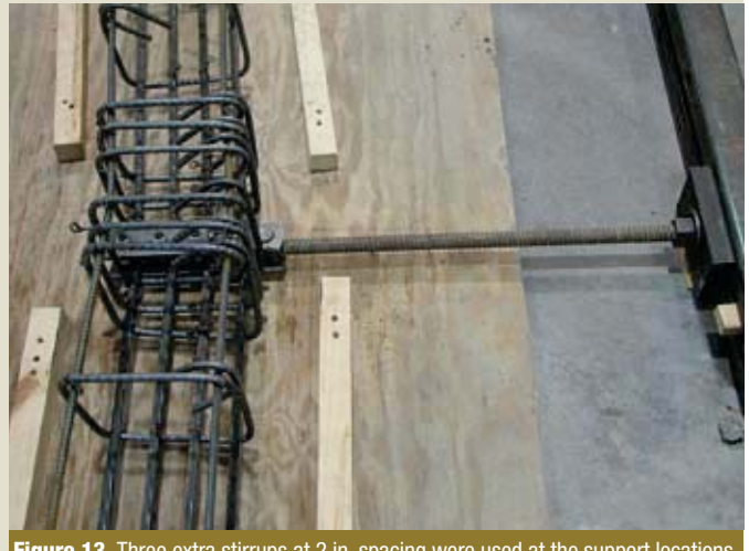
Figure 13. Three extra stirrups at 2 in. spacing were used at the support locations. Note: 1 in. = 25.4 mm.
