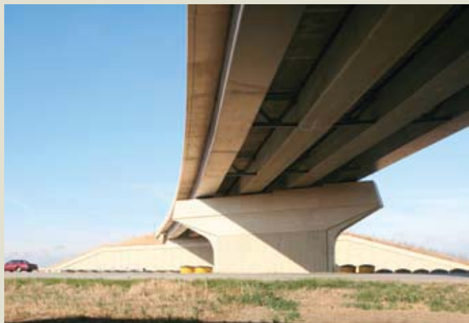
Figure 6. The Arbor Road Bridge in Lincoln, Neb., is a two-span, horizontally curved, precast concrete-girder bridge with a skew of 31 degrees and a central angle of about 3 degrees.
